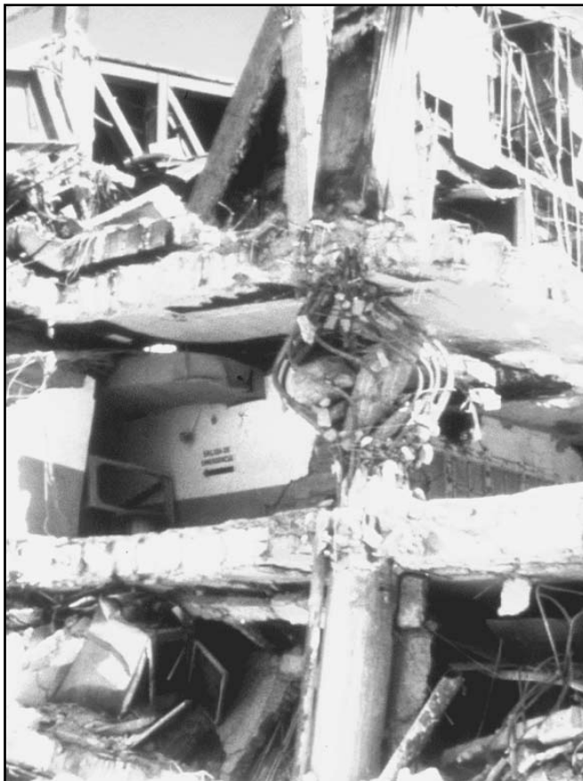
Figure 1 – Building collapsed due to an earthquake
